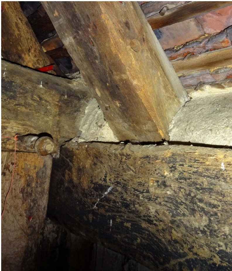
Figure 13. Rafter hole shown by a red pencil above the tie-beam and the rafter hole is seen in the foreground rafter. Photo taken in North Cray House, Weald and Downland Museum
