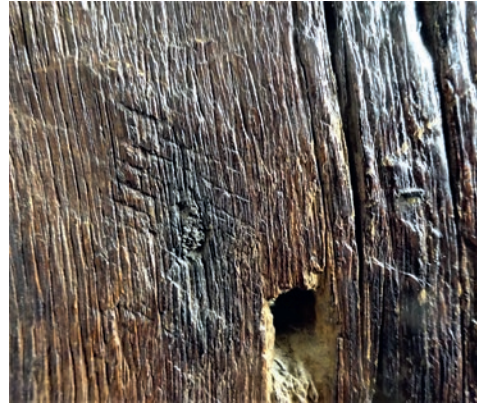
17 Saw marks missed by the finishing tool. Photo Paul Reed
